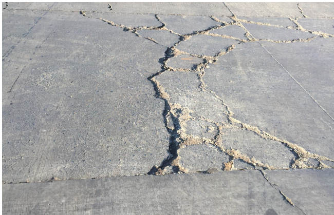
Hard Stand Damage
