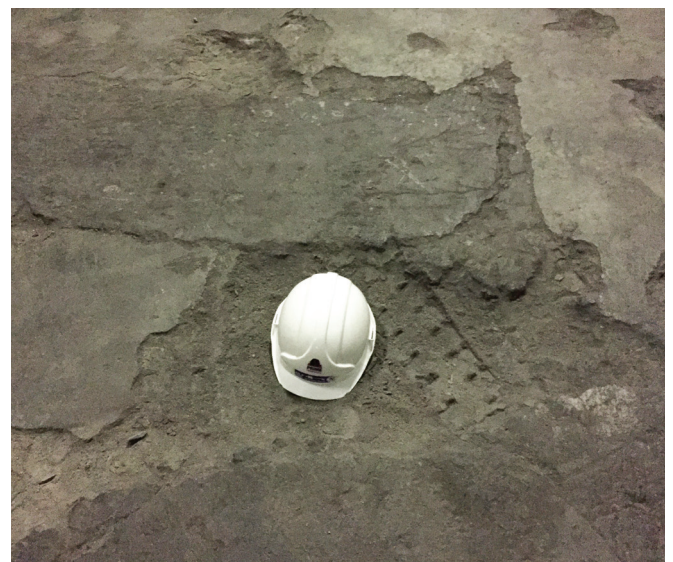
Floor surface failure
