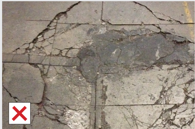
Joint damage without Mamba Joint.
